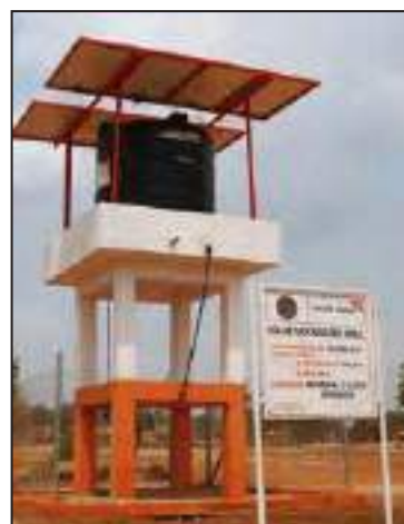
Solar powered mechanised borehole in Kenyasi No. 2
