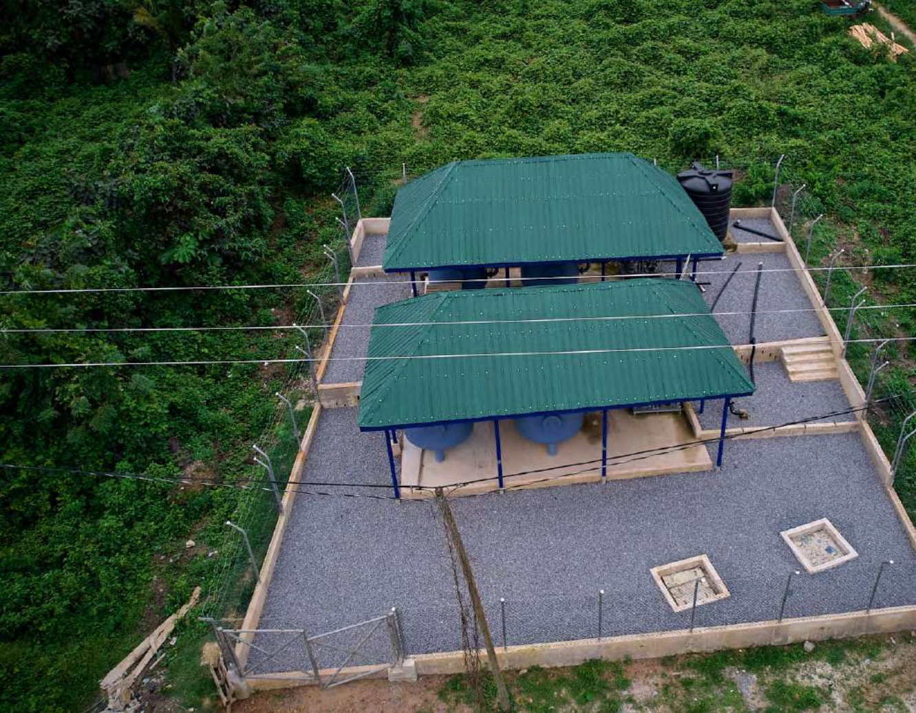
The new water system in Wassu Dunkwa
